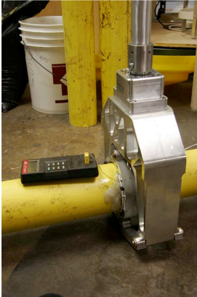
Figure 28: Overlapping full-wrap patch applied to 4" MDPE pipe during demonstration for Northwest Natural
