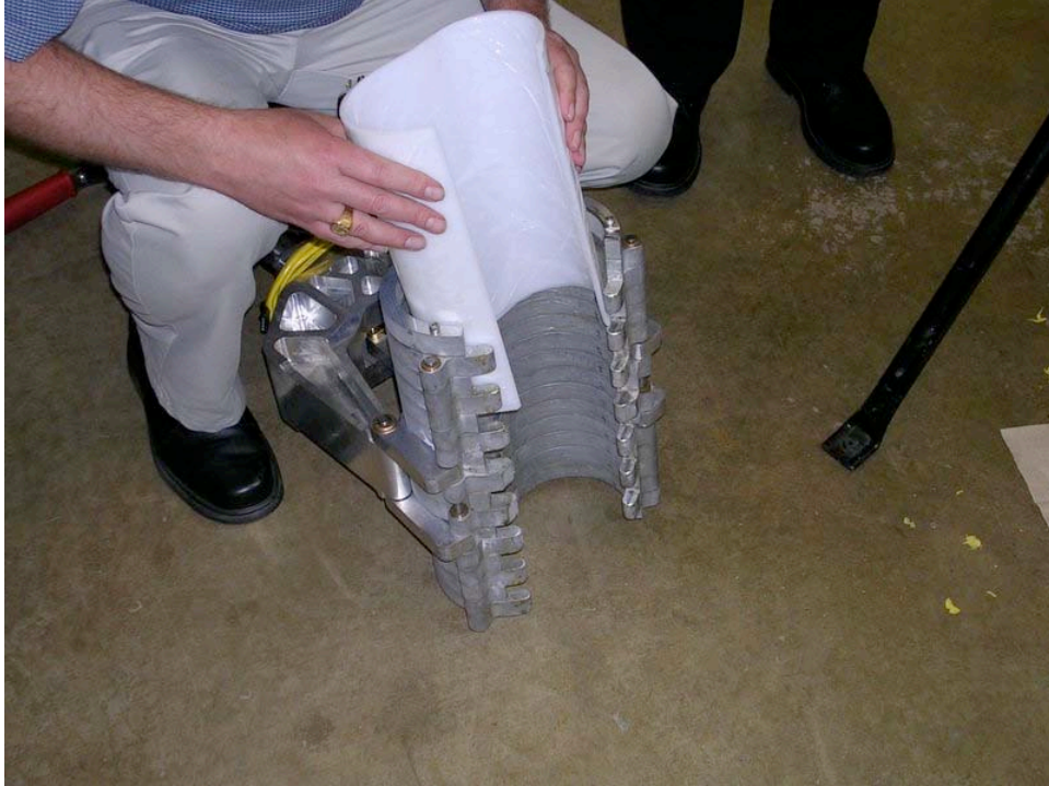
Figure 48: PE gel film repair patch being loaded into the engineer prototype at Nicor Gas demonstration in Naperville, IL
